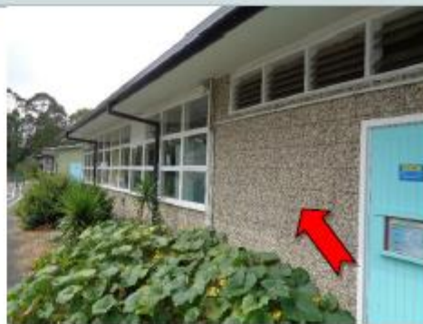
Photo 4 Block A, Ground Floor, External, walls, construction joint mastic to blockwork (Refer BJ0498) – Asbestos detected
