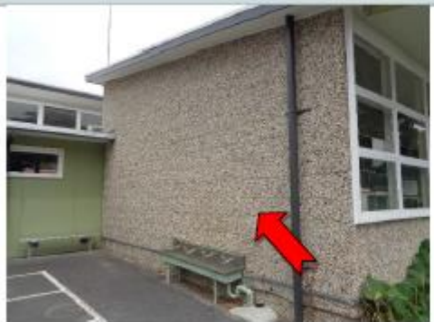
Photo 5 Block A, Ground Floor, External, walls, construction joint mastic to blockwork (Refer BJ0498) – Asbestos detected
