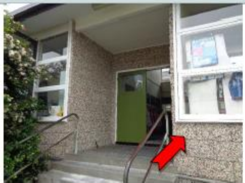
Photo 3 Block A, Ground Floor, External, walls, construction joint mastic to blockwork (Refer BJ0498) – Asbestos detected
