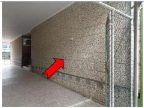
Photo 1 Block A, Ground Floor, External, walls, construction joint mastic to blockwork (Refer BJ0498) – Asbestos detected
