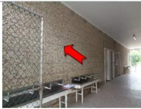
Photo 2 Block A, Ground Floor, External, walls, construction joint mastic to blockwork (Refer BJ0498) – Asbestos detected
