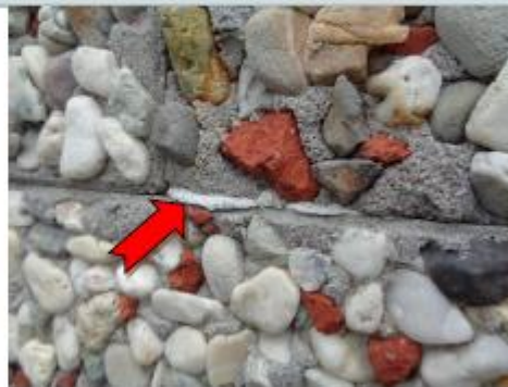
Photo 6 Block A, Ground Floor, External, walls, construction joint mastic to blockwork (Refer BJ0498) – Asbestos detected
